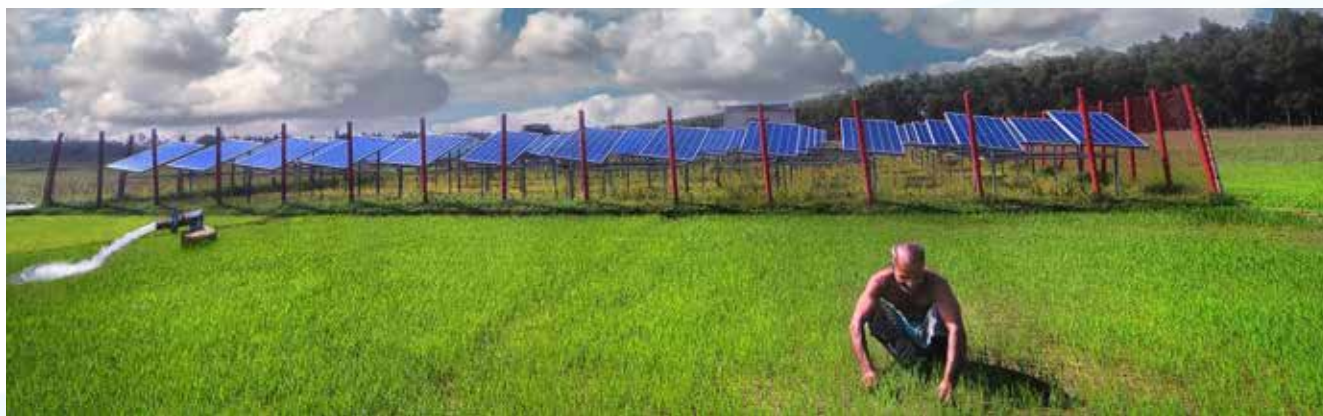
Solar powered Irrigation Systems ( http://idcol.org/home/solar_ir )
